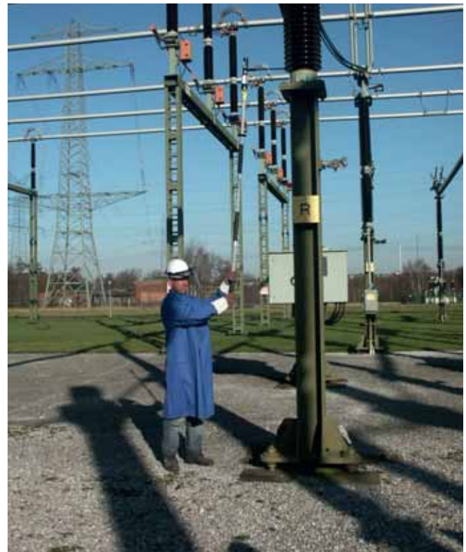
Use of an ASP distance voltage detector in an outdoor switching station
