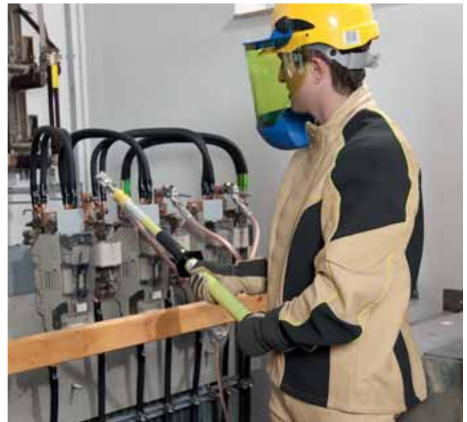
Attaching an earthing and short-circuiting device using adequate personal protective equipment
