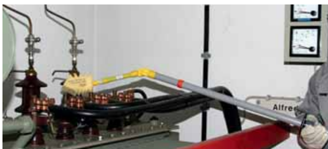
TFRS MS combined cleaning kit used for dry and damp cleaning of a transformer under live conditions
