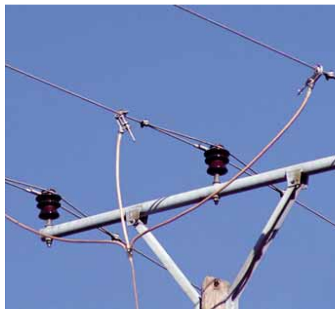
Phase screw clamps used on an overhead line
