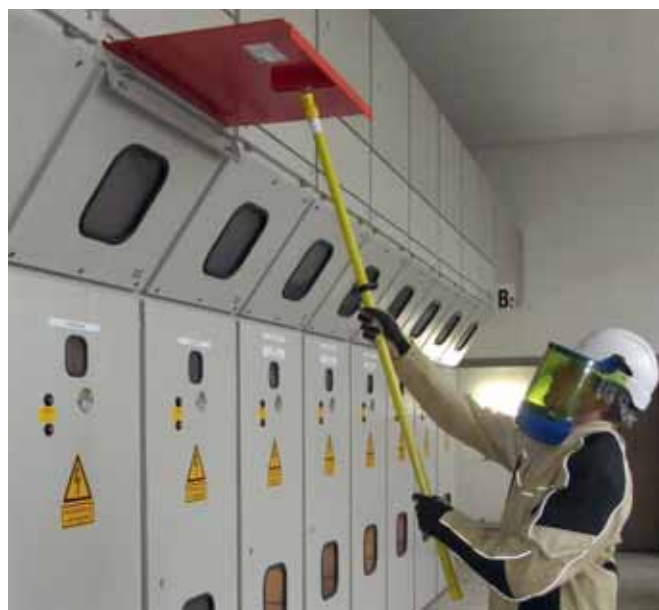
Inserting an insulating protective shutter (type A3) by means of an operating stick
