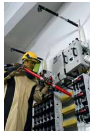
Figure 3: Work on an open switchgear installation using a mobile arc fault protection system.
