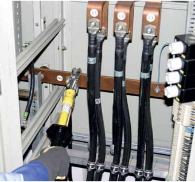
Attaching an earthing and short-circuiting device in a low-voltage switchgear installation using an earthing handle.
