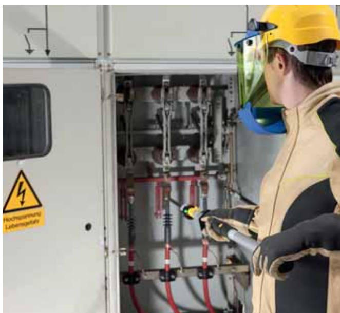
PHE III voltage detector with visual and acoustic indicator used for an indoor switchgear installation
