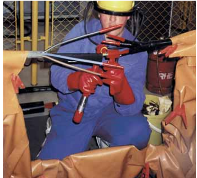
Covering live parts
