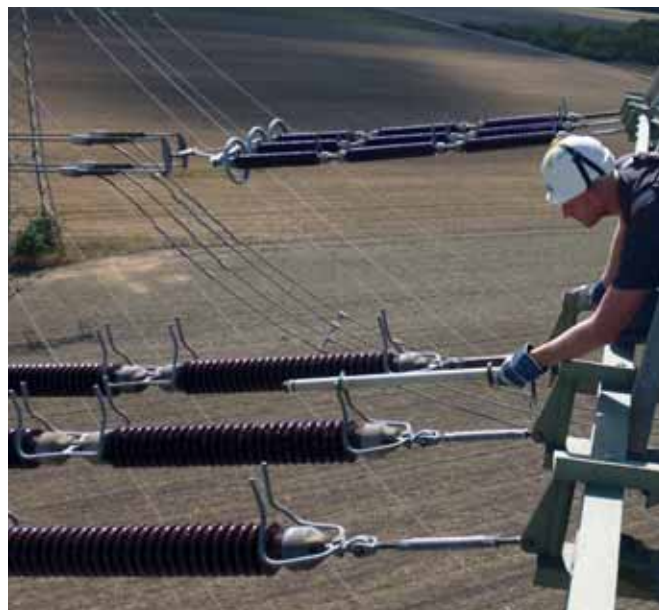
High-voltage indicator used on a 110 kV overhead line.
