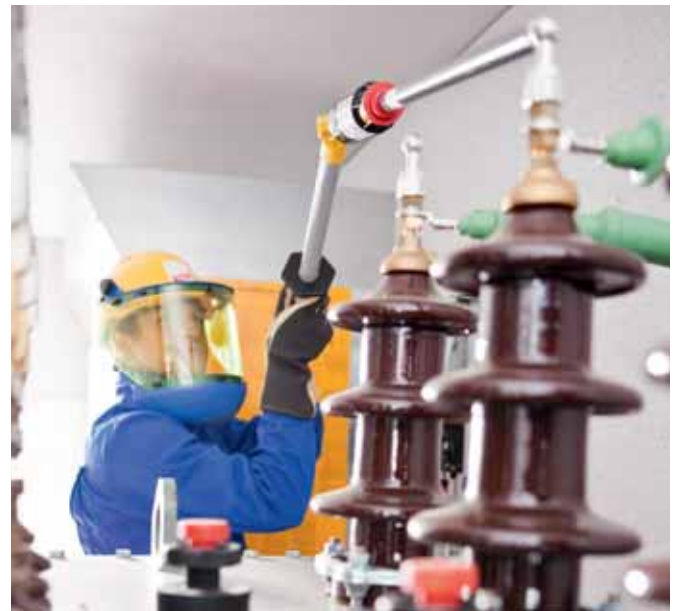
PHE III indicator with test prod, universal gear coupling and insulating stick
