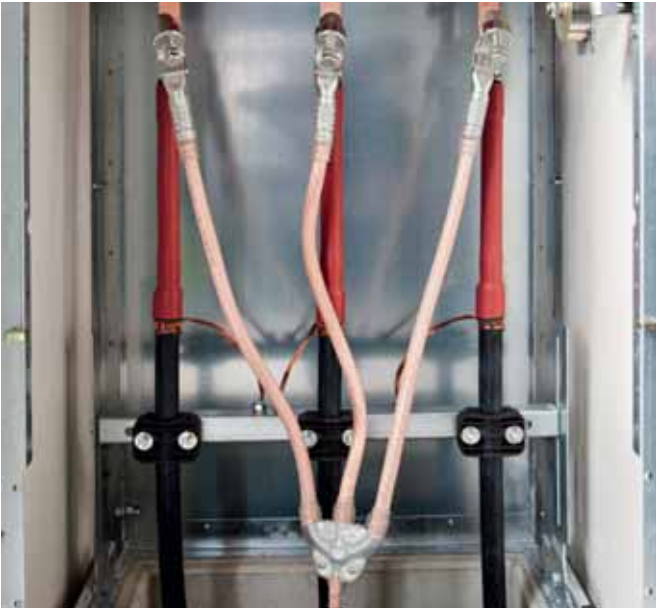
Equipped three-pole earthing and short-circuiting device in a switchgear installation
