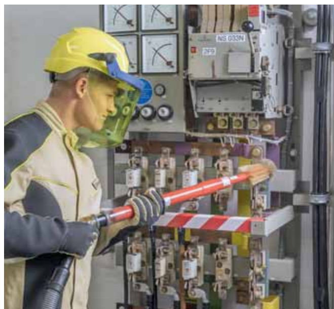
Live cleaning of a low-voltage switchgear installation using the TRS NS dry cleaning kit
