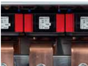
Built-in protection transformers
