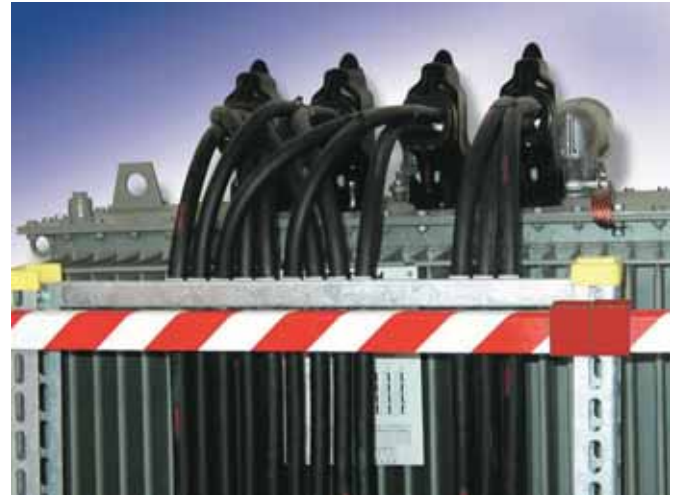
Barrier in a transformer station.
