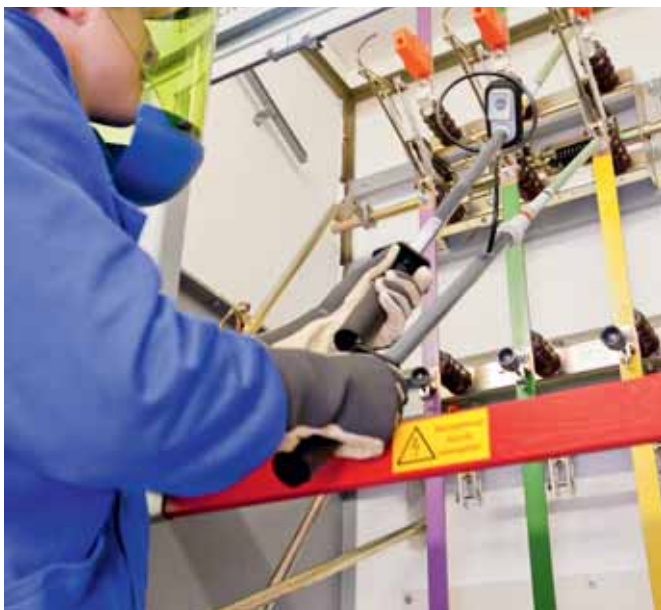
Two-pole PHV phase comparator with a pair of green test prods (15 ... 24 kV) used in a 20 kV switchgear installation
