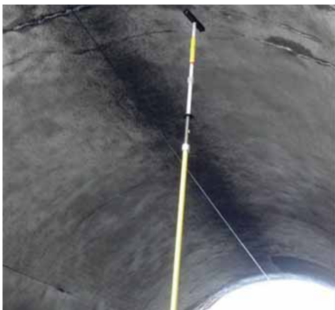
Removing icicles on a tunnel entrance.
